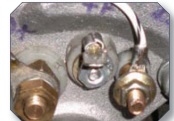
Close up view of the three terminals, New IF terminal without a wire lead yet.
