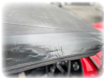
Inventive way to fix a hood. Duct tape and staples. Why spend the money for a hood used once every 5 years?
